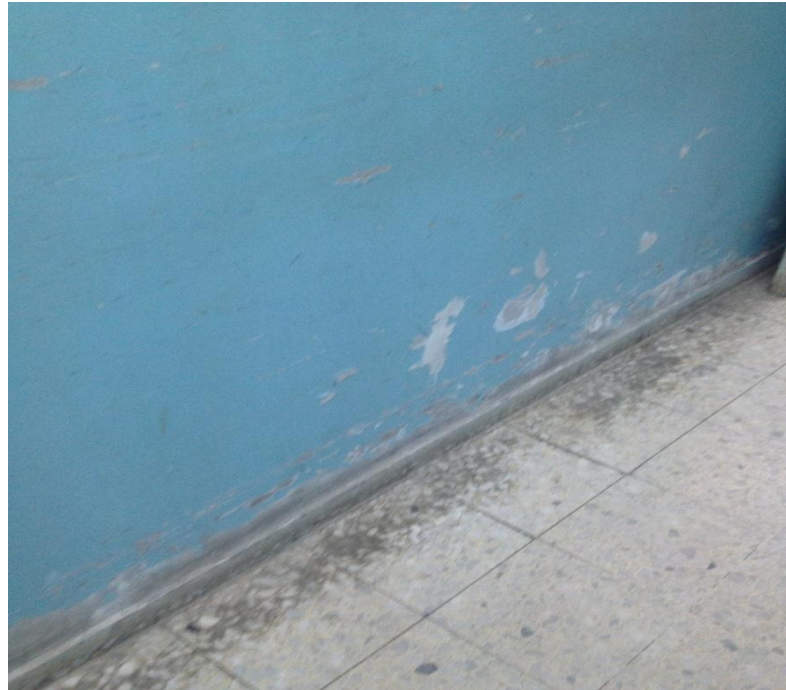
Figure 4.14 Wet areas problems in floors and walls.
