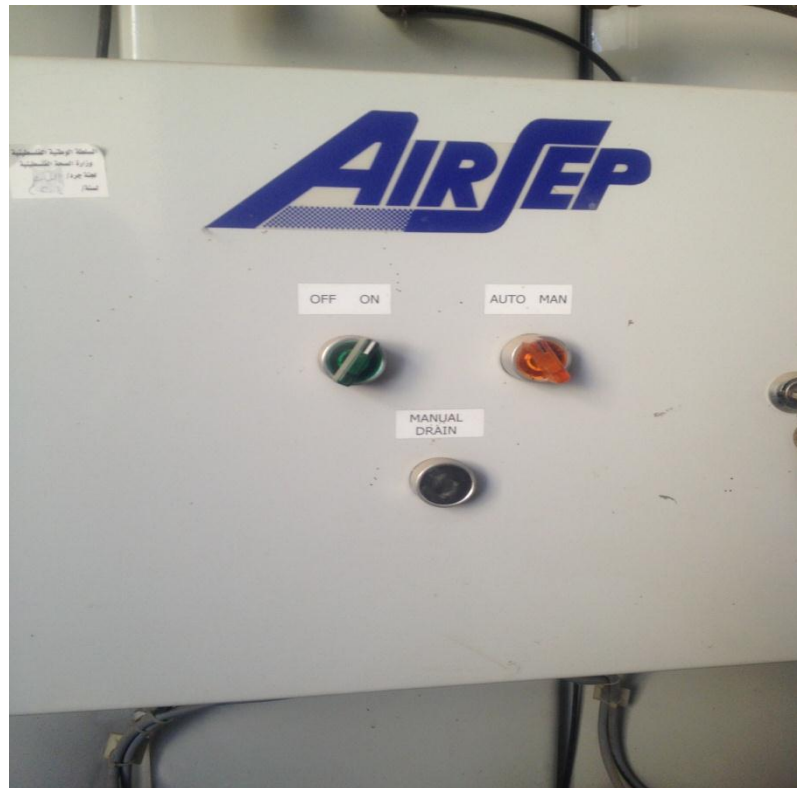
Figure D.6 Medical gasses station
