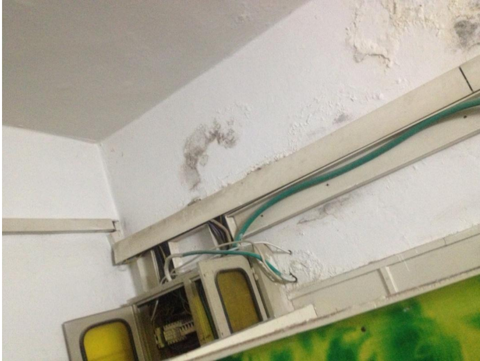
Figure D.5 Moisture in walls
