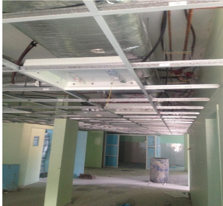
Figure 4.18 Medical gazes installation in ceilings
