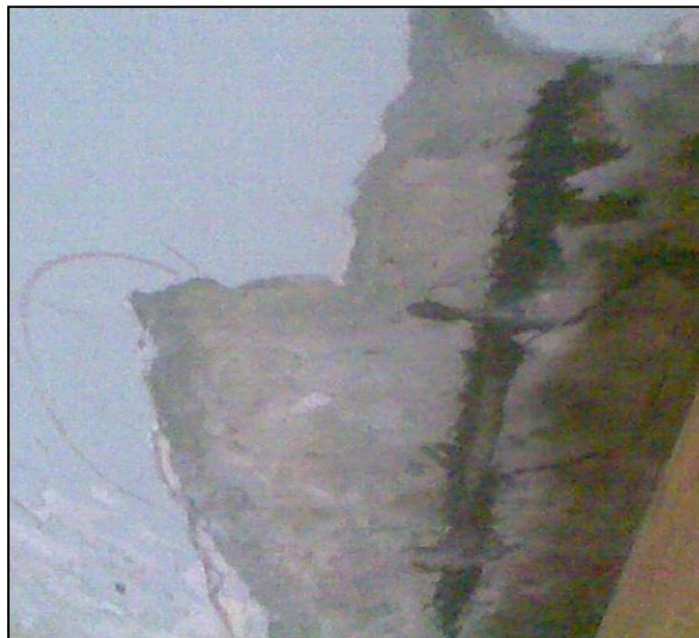
Figure.4.20 Erosion appears in the column
