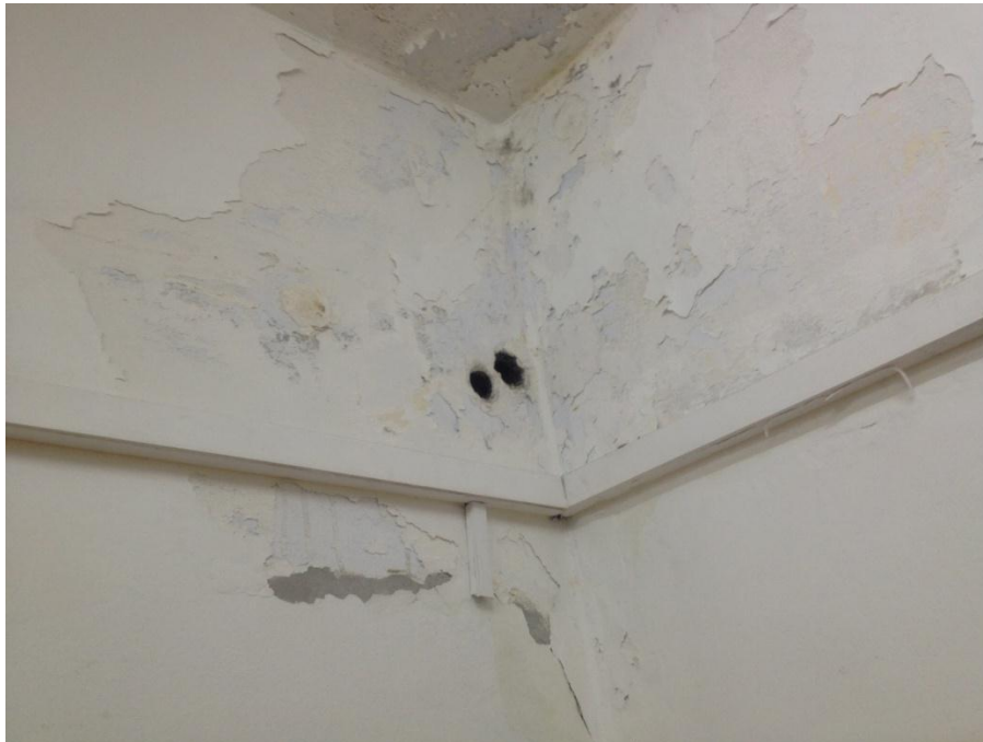
Figure D.4 Moisture in walls
