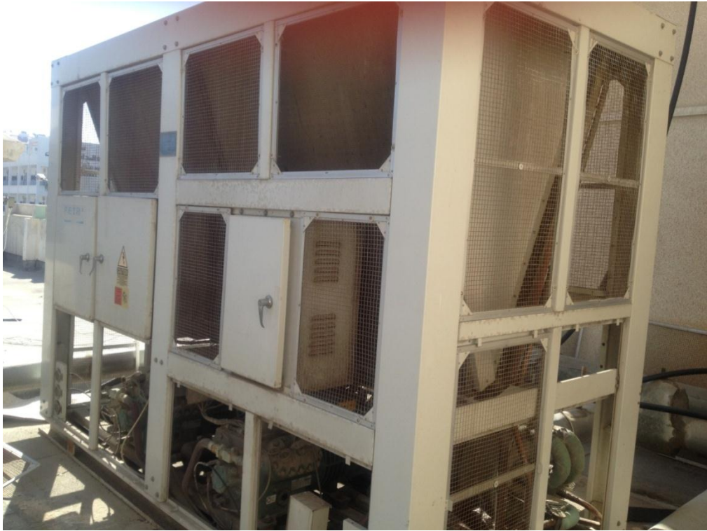
Figure D.9 chillers
