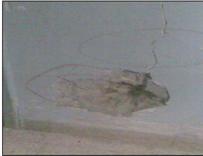
Figure 4.19 Deep cracks in the walls
